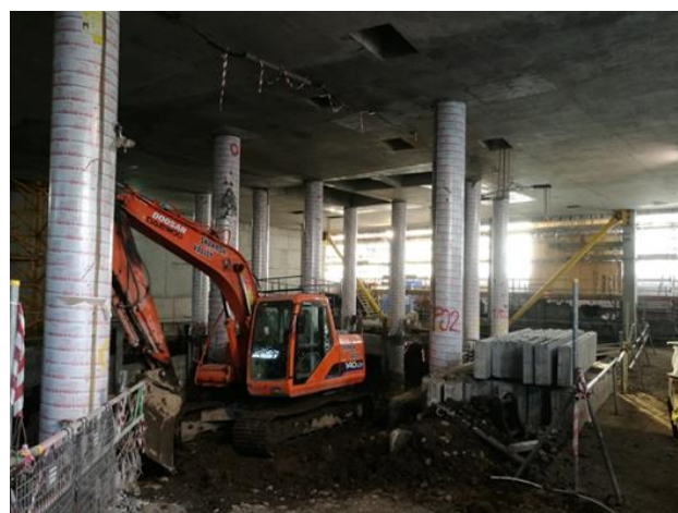
Figure 5. Image showing Level 1 transfer slab supported by pile-columns, RC walls and temporary stability bracing.
